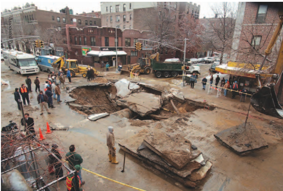
Emergency construction crews examine a ruptured water main in Queens, New York City, January 3, 1996.
