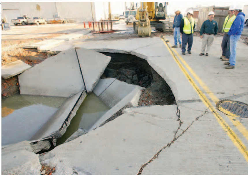
A water main break in Gillette, Wyoming in August 2006. About 3 million gallons of water erupted causing at least $100,000 in repairs and requiring traffic diversions.
