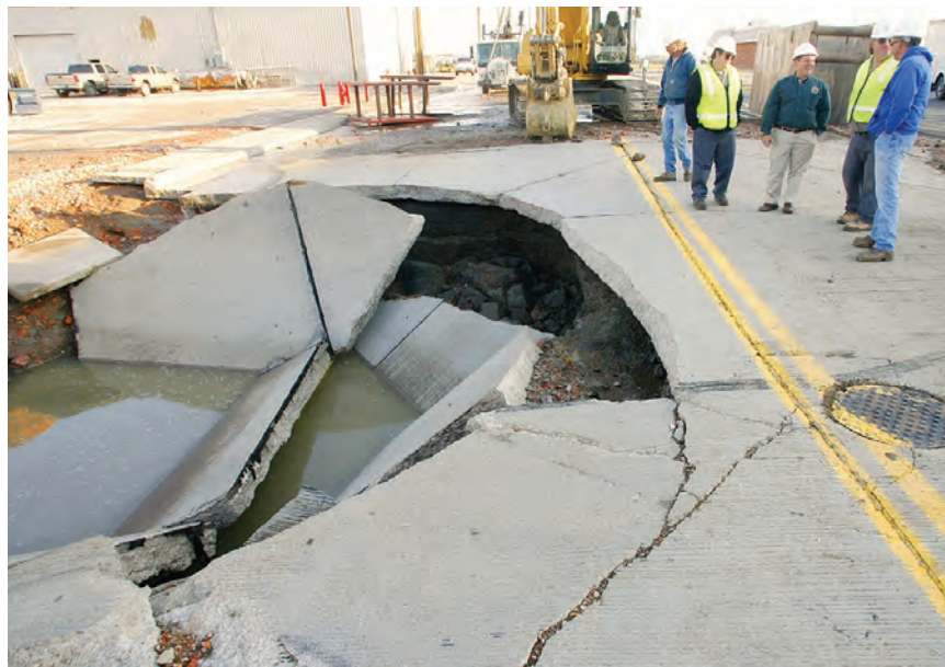
A water main break in Gillette, Wyo. in August 2006. About 3 million gallons of water erupted causing at least $100,000 in repairs and requiring traffic diversions.
