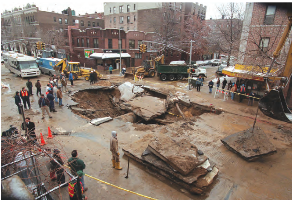
Emergency construction crews examine a ruptured water main in the Queens Borough of New York January 3, 1996.
